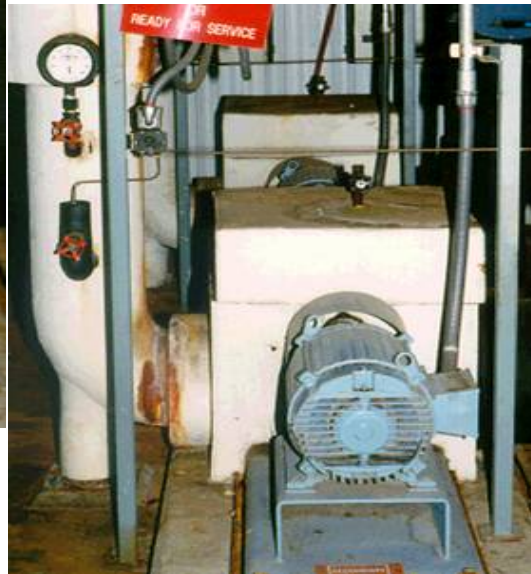
Combined motor & pump efficiency = 59%
